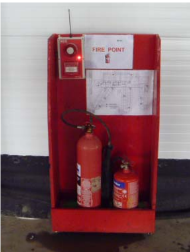
A WES equipped fire point at Dunfermline High School
